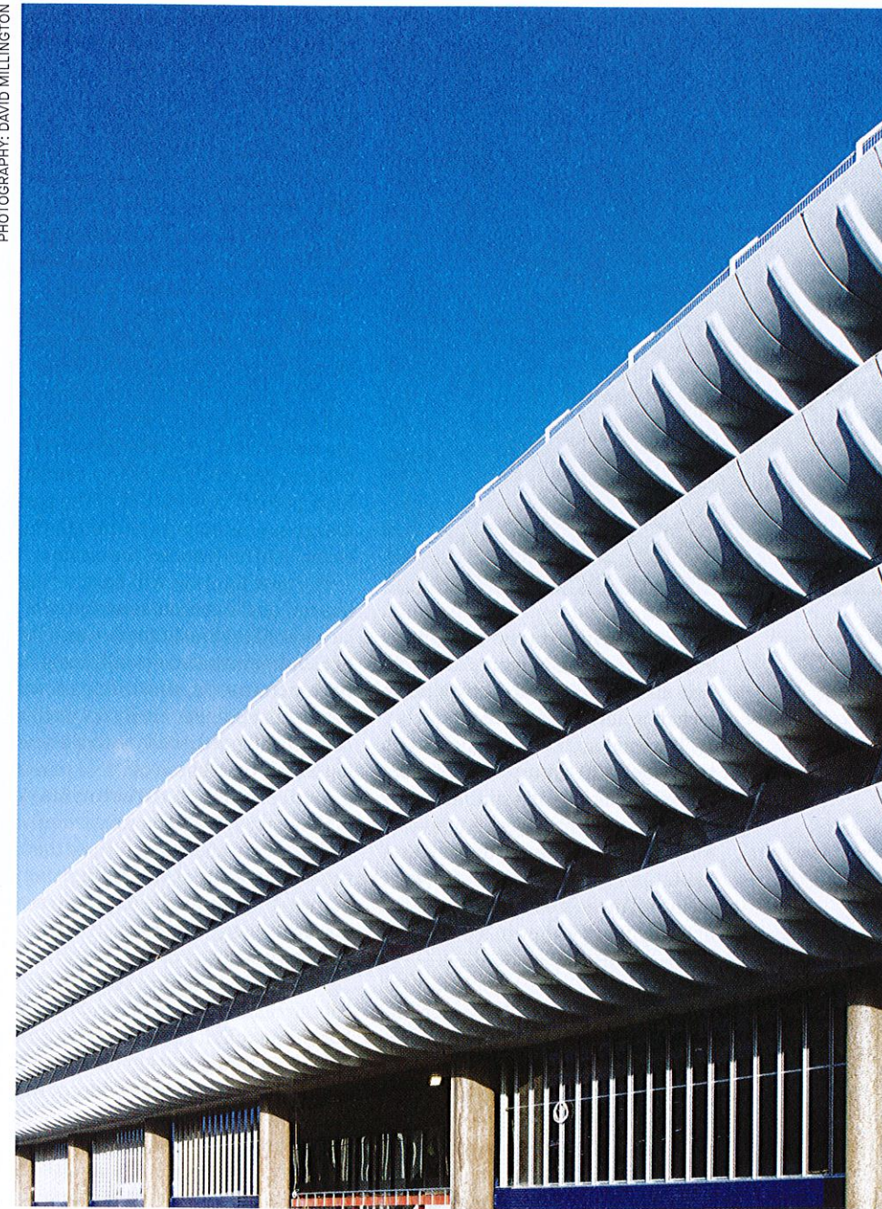
The distinctive scallop shell facade of the bus station has been restored and treated with anti-carbonation paint
