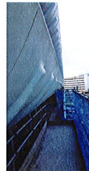
Conlon and concrete repairs contractor Makers devised a bespoke cantilevered cradle to access the scallops
