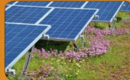
COMPLETED PHOTOVOLTAIC GREEN ROOF
