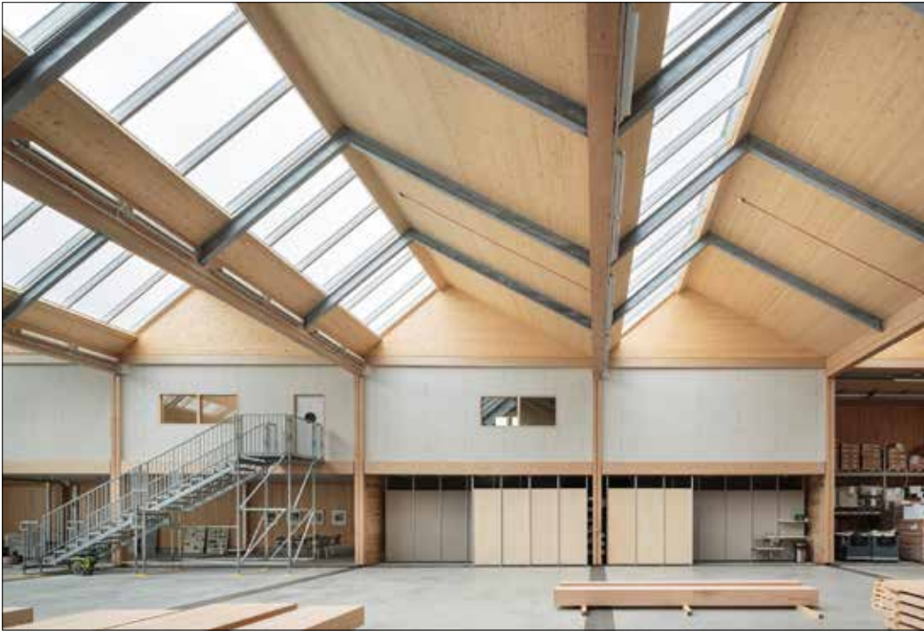
Left The Velux skylights were positioned at 40 degrees to maximise north light
